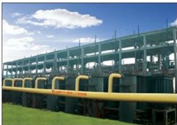
Two Stage Coal Gasifier Cold Gas Station
